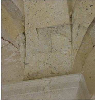
Crushing / shearing of brackets
